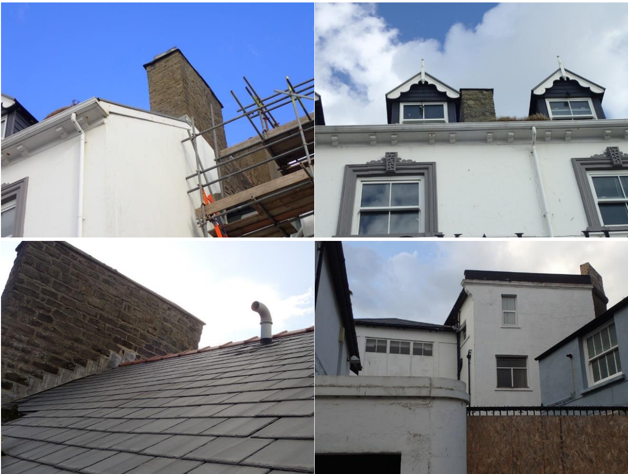
External photographs (clockwise from top-left): southern gable end; upper front (west) face; rear of building; eastern roof section
