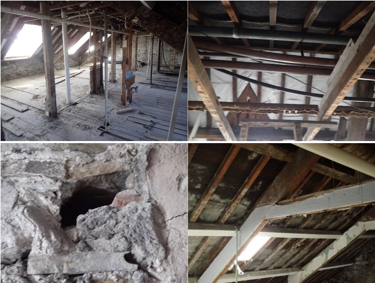
Internal photographs (clockwise from top-left): Upper storey; ridge showing newer (white) membrane and older (black) bitumen membrane; minor cavity in internal gable-end wall
